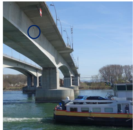
Fig.1 Photo of the Rhine bridge in Worms. The inlet position is indicated by a blue circle.
