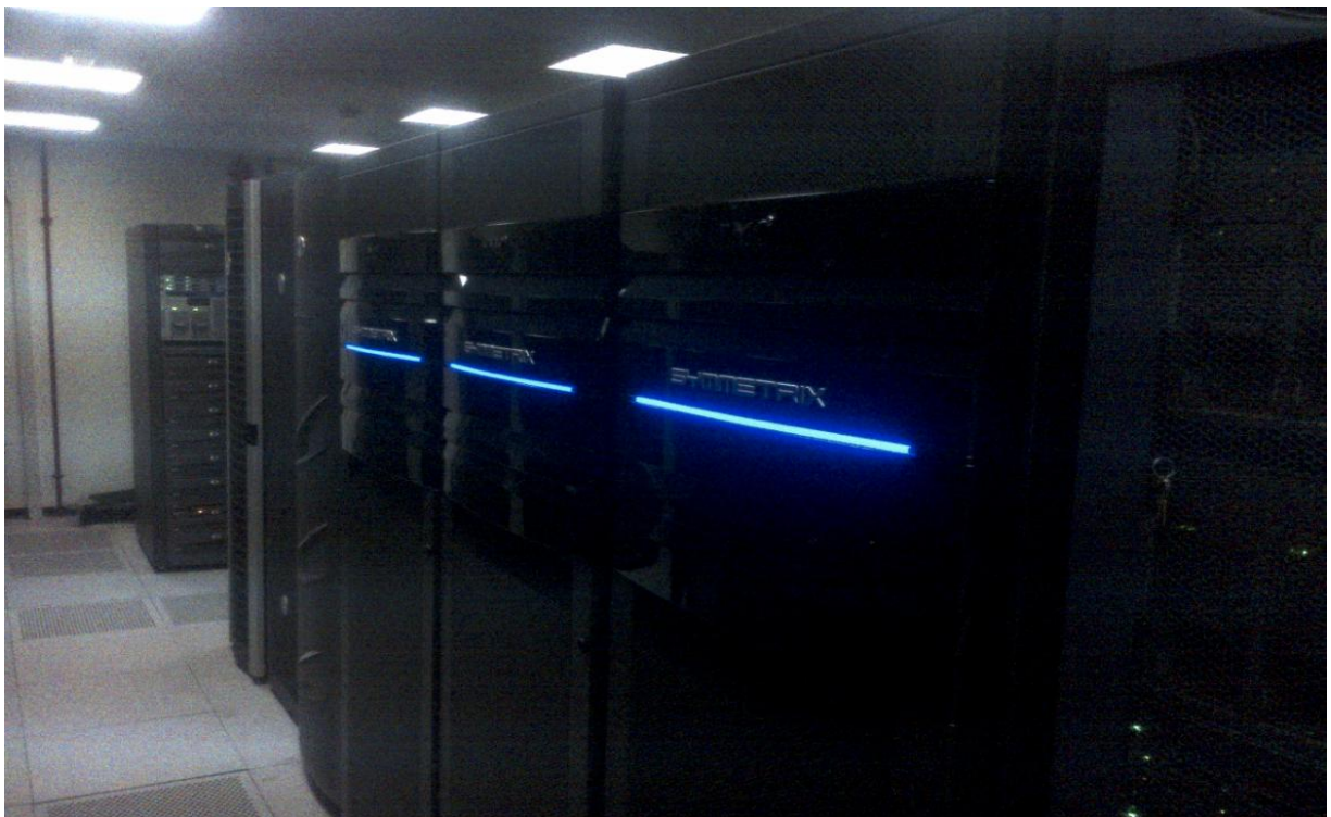
A photograph of the computer server room in ADPF
