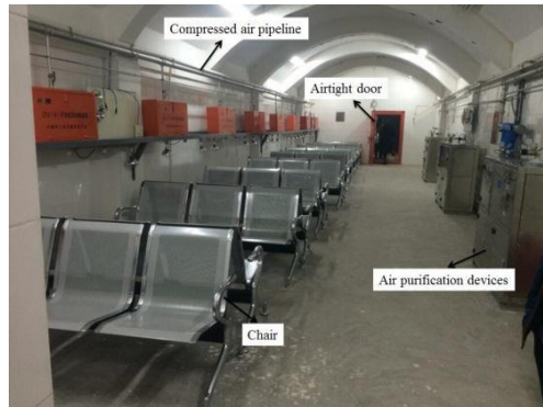
Fig. 1. Interior of a typical permanent refuge chamber.
