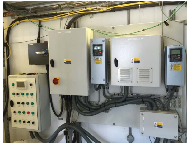
System Control Panel
