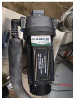
(b) Water circulating pump
