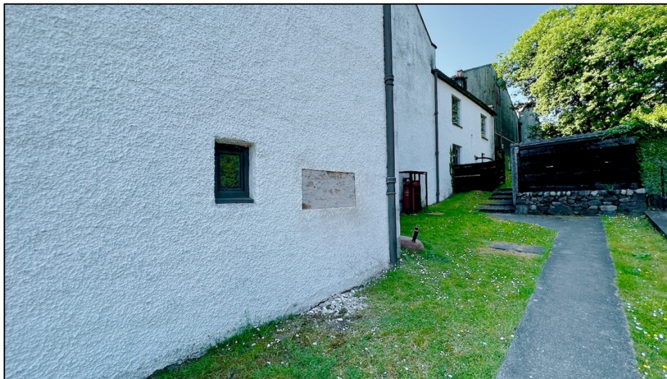
Figure 22: The building, aspect, and location of the experimental wall section. The section is north-east facing. The top layers of concrete were removed from the wall section, exposing the original stone beneath prior to the application of new lime render
