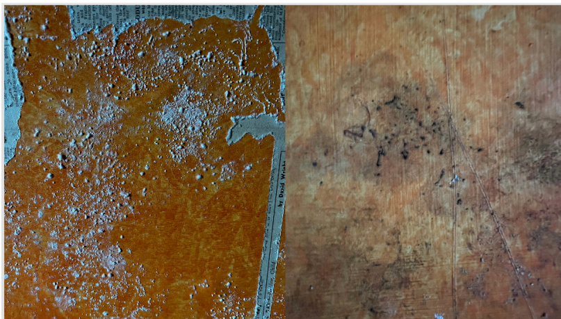
Figure 50: Samples of mould collected from damp surfaces of interior walls. White mould, situated on damp wallpaper (left of image), was identified as the source of a distinctive odour, commonly accompanied by a confluence of mould species such as Cladosporium , Penicillium , and Aspergillus . On the right, the presence of black mould exemplifies Stachybotrys proliferation. The images illustrate the manifestation of mould growth on
