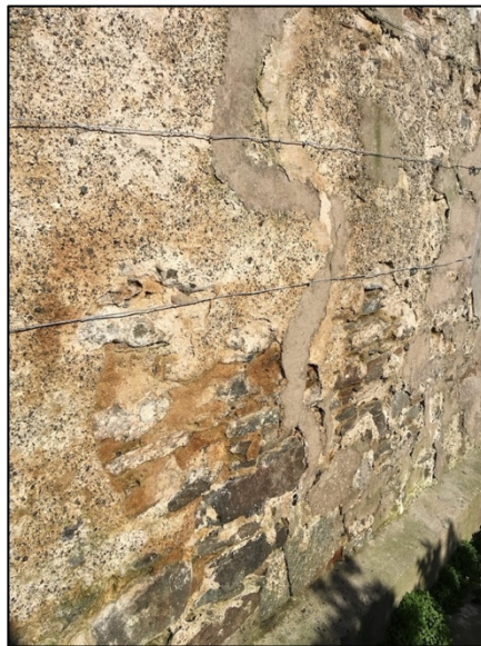
Figure 6: Photograph illustrating the insertion of lime and concrete into stonework in a weather-exposed wall section in the Northern Isles, Scotland. Original protective limewash coatings have eroded leaving underlying lime render exposed. Weathering and trapped moisture has resulted in render loss and the formation of large cracks as a result of the introduction of concrete. The imbalance between the lime and concrete traps moisture resulting in an uneven erosion of lime and delamination of the stone surface. (Image source: author)
