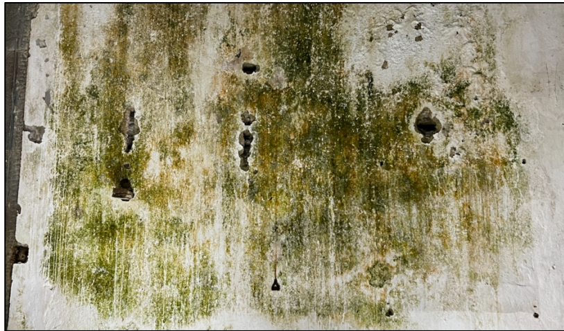
Figure 46: Penicillium chrysogenum growing on an internal plaster wall in a damp environment in a heritage-at-risk building in Scotland. It reproduces through spores or conidia which are carried by air currents to new damp colonisation sites in the building. The airborne spores are implicated as human allergens due to the presence of serine proteases as major allergenic proteins. (Author's image)
