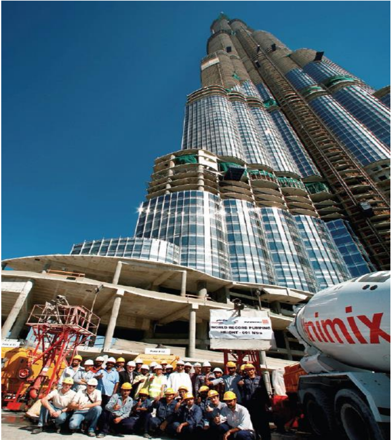
Figure 5-63 World record concrete pumping height of 601 m was achieved on 8 November 2007 (Aldred 2010)
