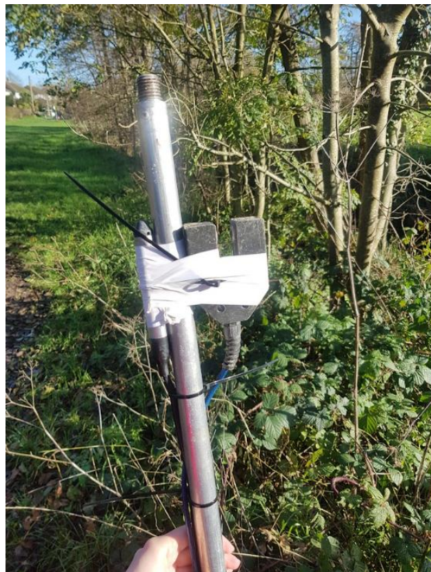
Figure 4. 1: Above: The wiring of the CR10x gauging station at Drop Lane with the pressure, conductivity and water temperature and turbidity sensors plugged in. Below: The stage and turbidity sensors secured to the metal pole using zip ties and tape, with the wiring directed and secured along the poles to the box (25 th November 2022).
